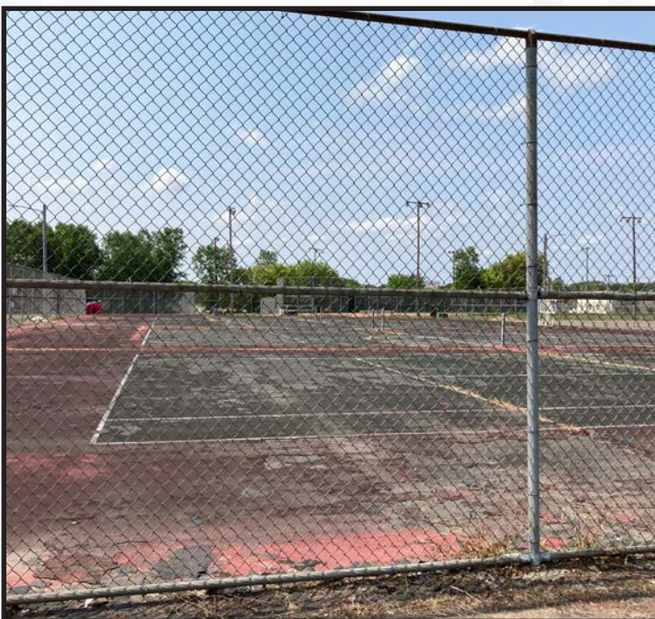
Tennis courts in poor condition
