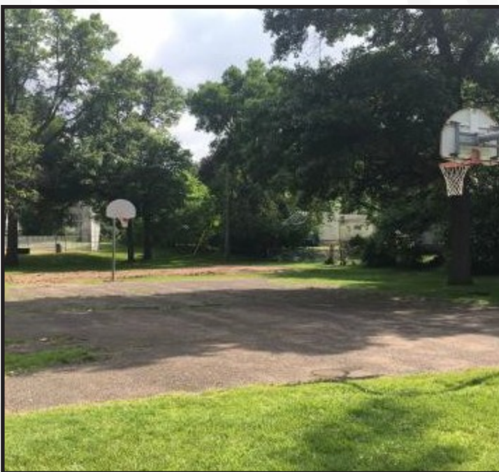
Basketball Court in poor condition
