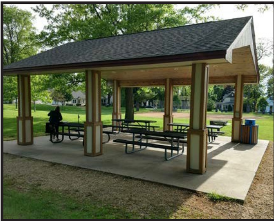
Shelter replaced in 2012
