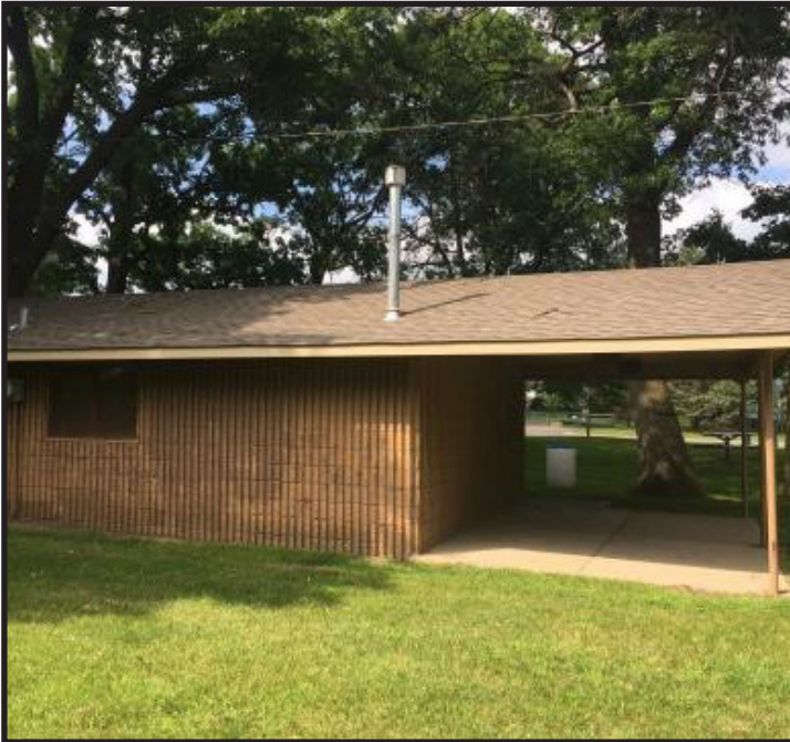
Building is at end of useful life
