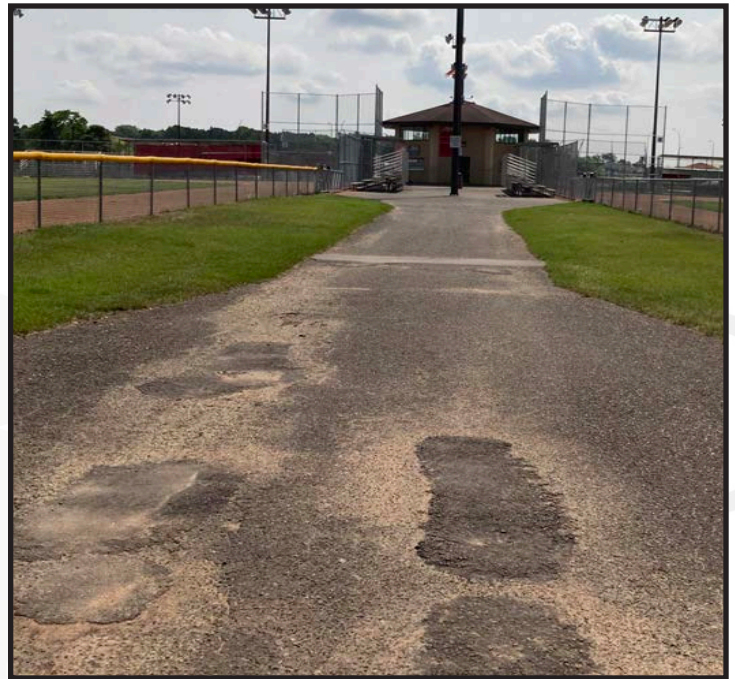
Concession stand and poor trail conditions
