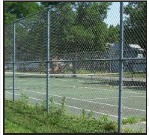
Tennis court in poor condition and is undersized
