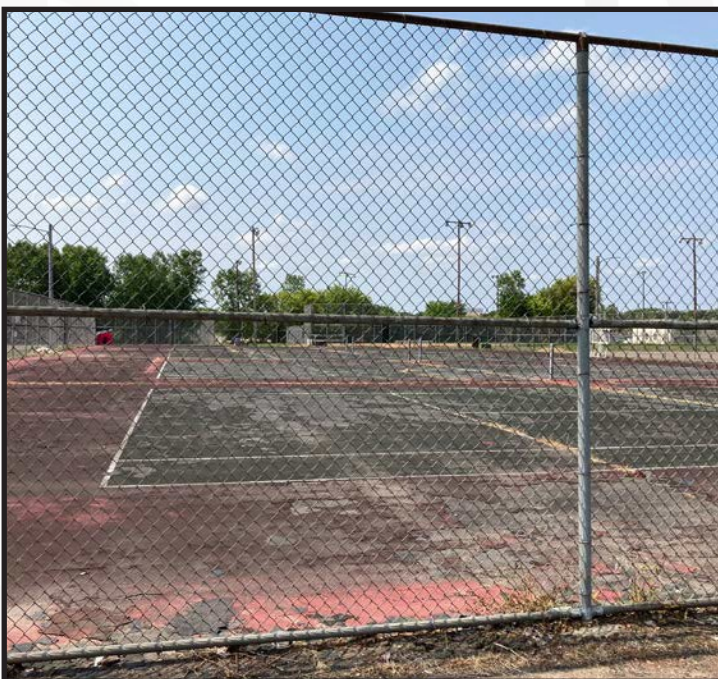
Tennis courts in poor condition
