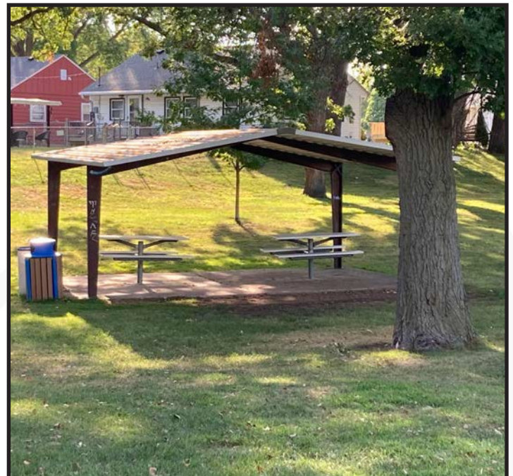
Shelter is at end of useful life
