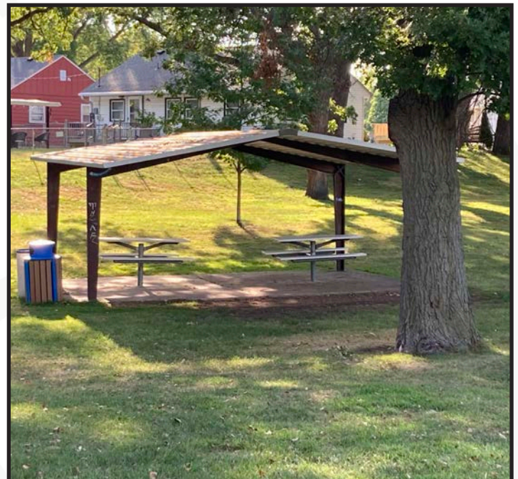
Shelter is at end of useful life
