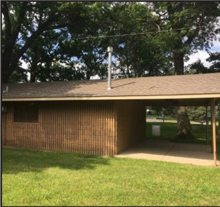
Building is at end of useful life
