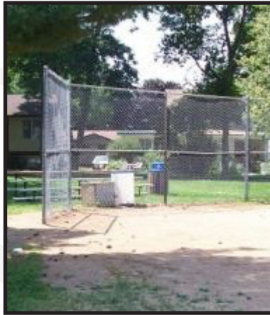
Ball field needs improvements
