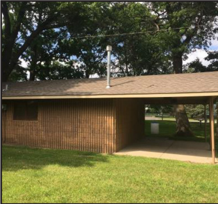
Building is at end of useful life
