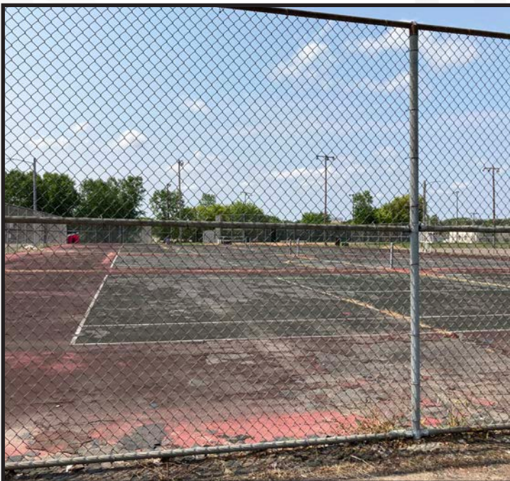
Tennis courts in poor condition
