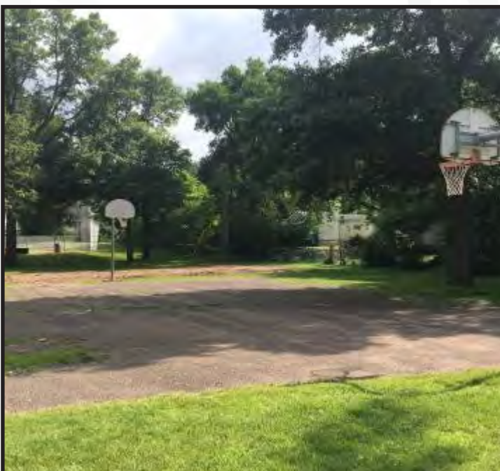
Basketball Court is in poor condition
