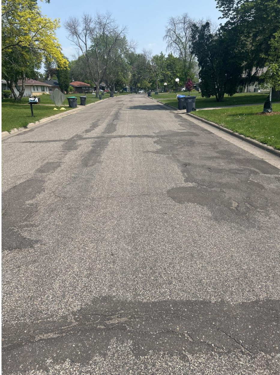
Shoshone Road 61.001, PCI = 52
