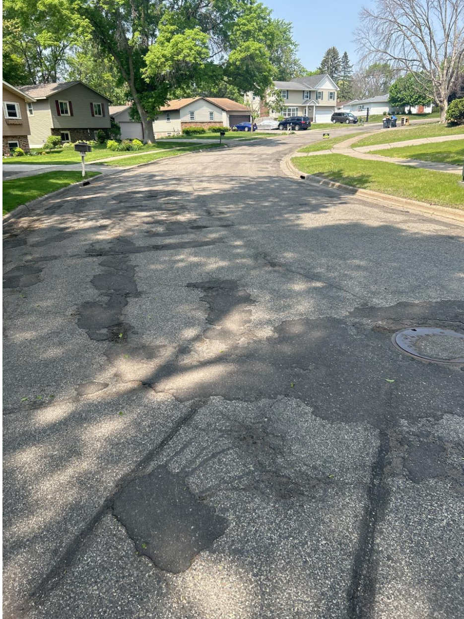
Buhl Avenue 7.001, PCI = 44
