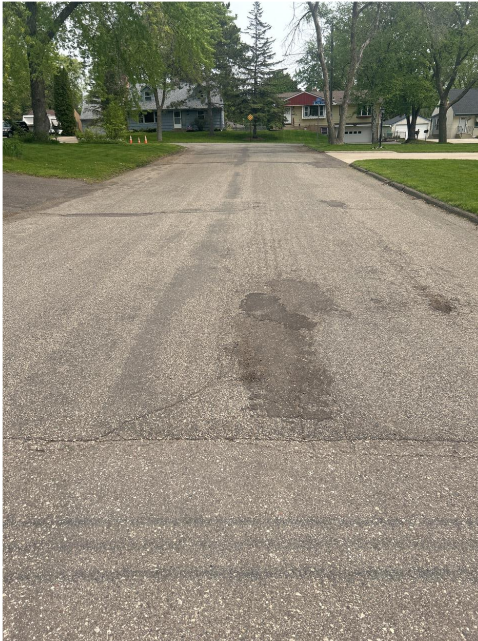
Shoshone Road 61.002, PCI = 59
