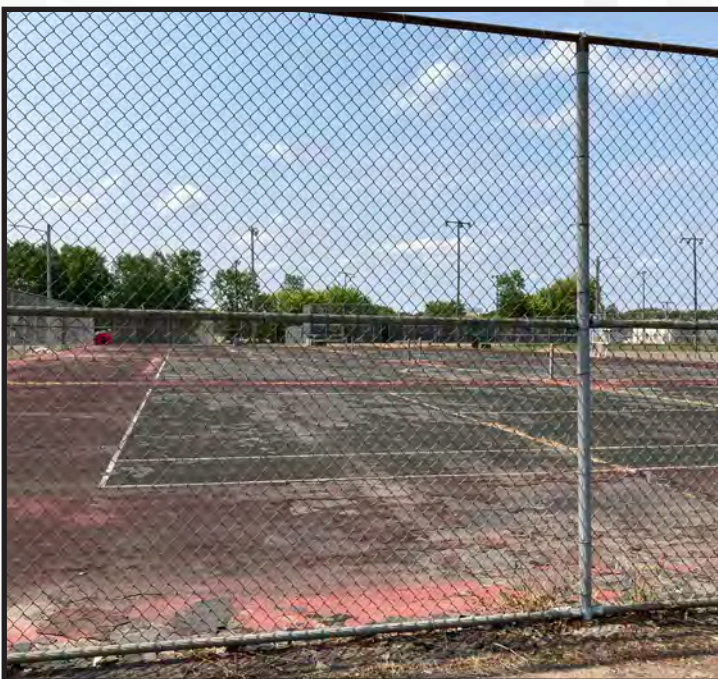
Tennis courts in poor condition
