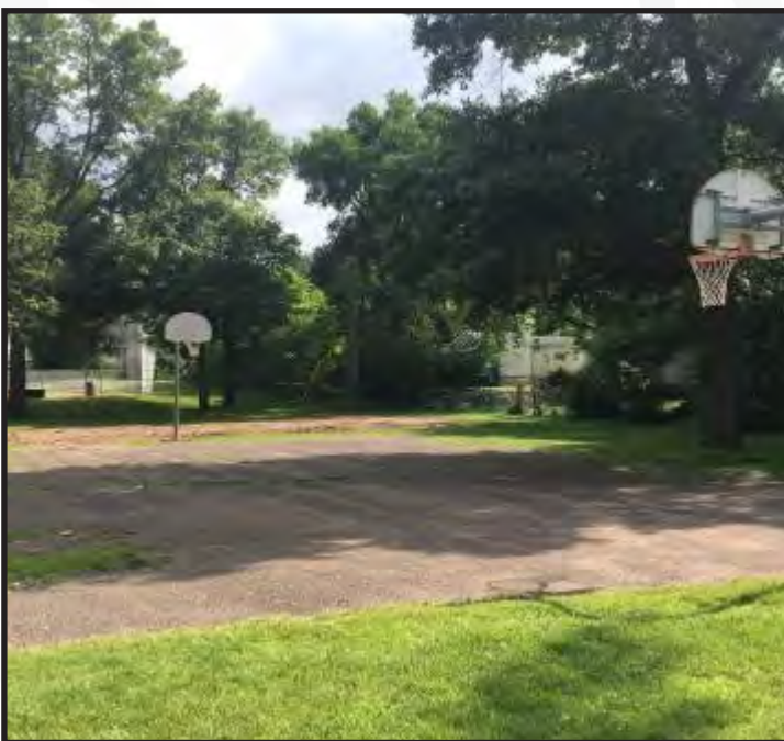
Basketball Court is in poor condition
