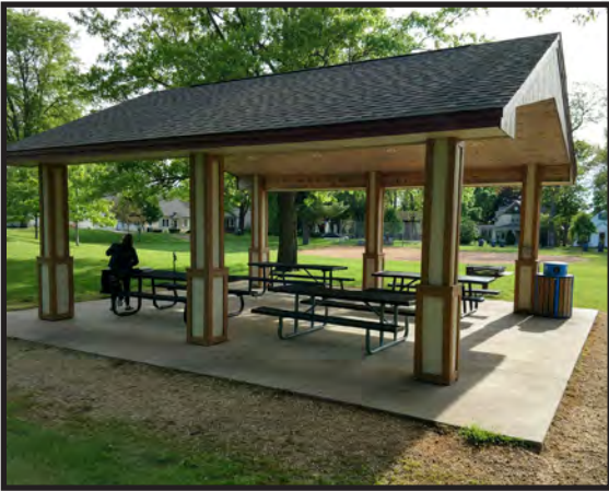
Shelter replaced in 2012; not connected by accessible walks
