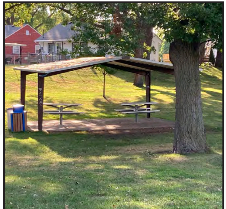
Shelter is at the end of its useful life
