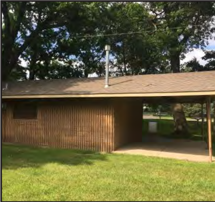
Building is at the end of its useful life
