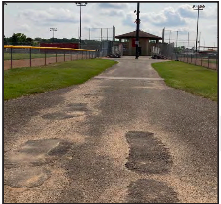
Concession stand and poor trail conditions
