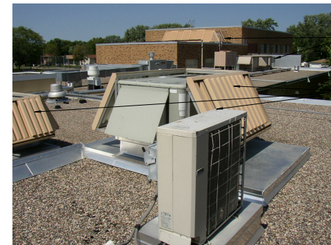
VIEW 2: EXISTING ROOF TOP EQUIPMENT
