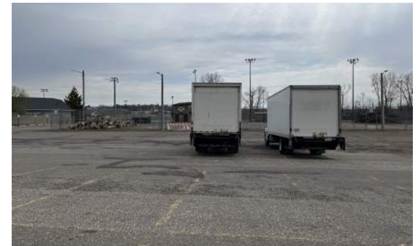
C - Parking lot in very poor condition
