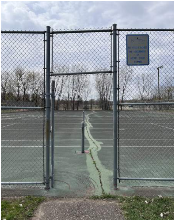
B - Unused tennis courts in disrepair
