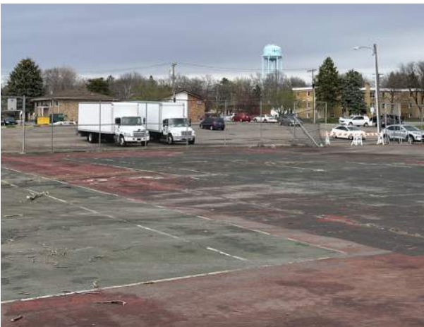
E - Unused tennis courts in disrepair
