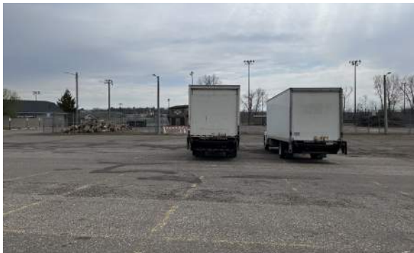
C - Parking lot in very poor condition
