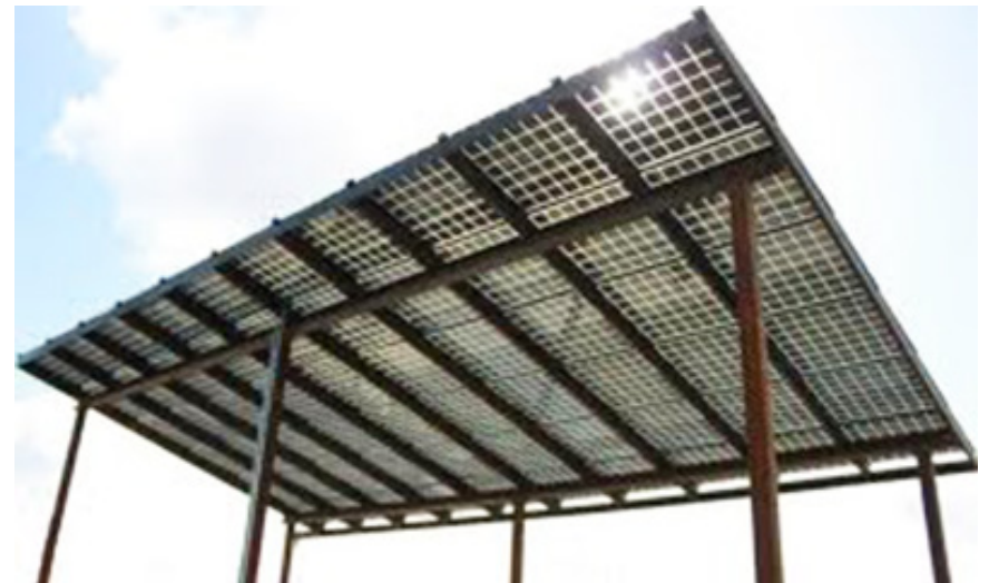
Solar Panels on Roof
