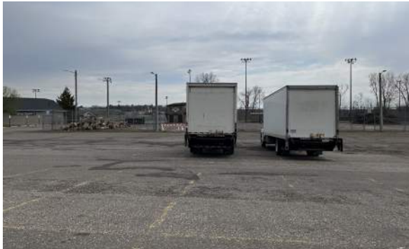
C - Parking lot in very poor condition
