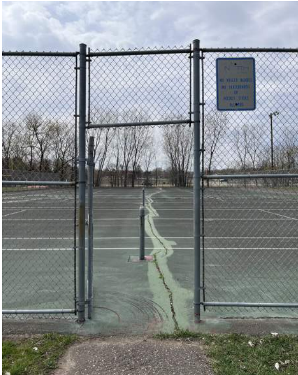
B - Unused tennis courts in disrepair
