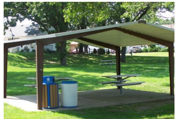
Shelter is recommended for replacement
