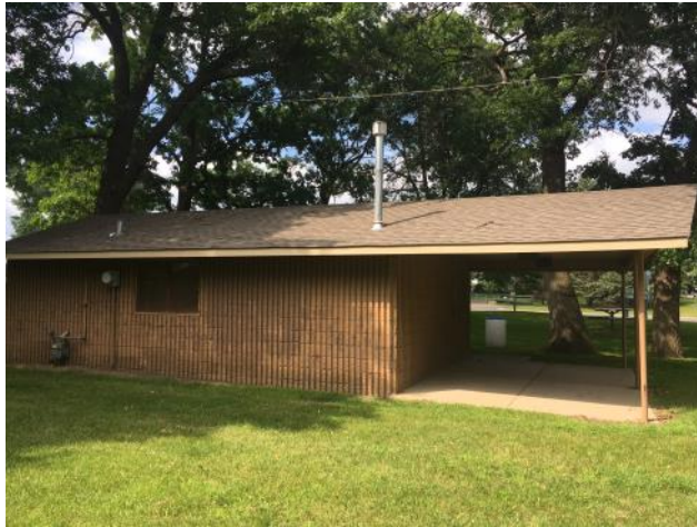
Building is recommended for replacement
