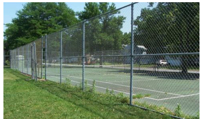
Tennis court needs resurfacing
