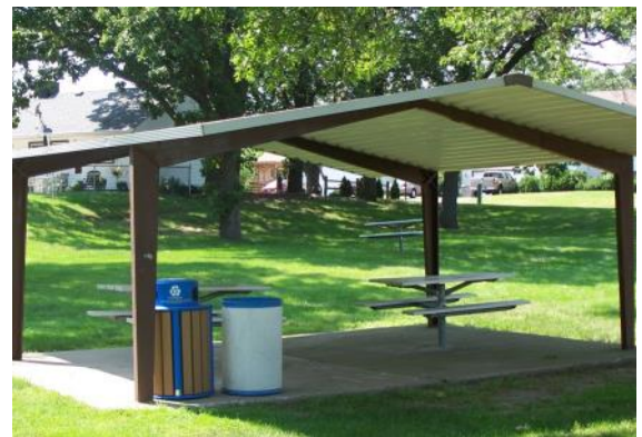
Shelter is recommended for replacement
