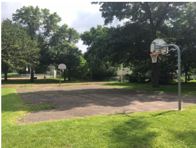
Basketball Court resurfacing is recommended.
