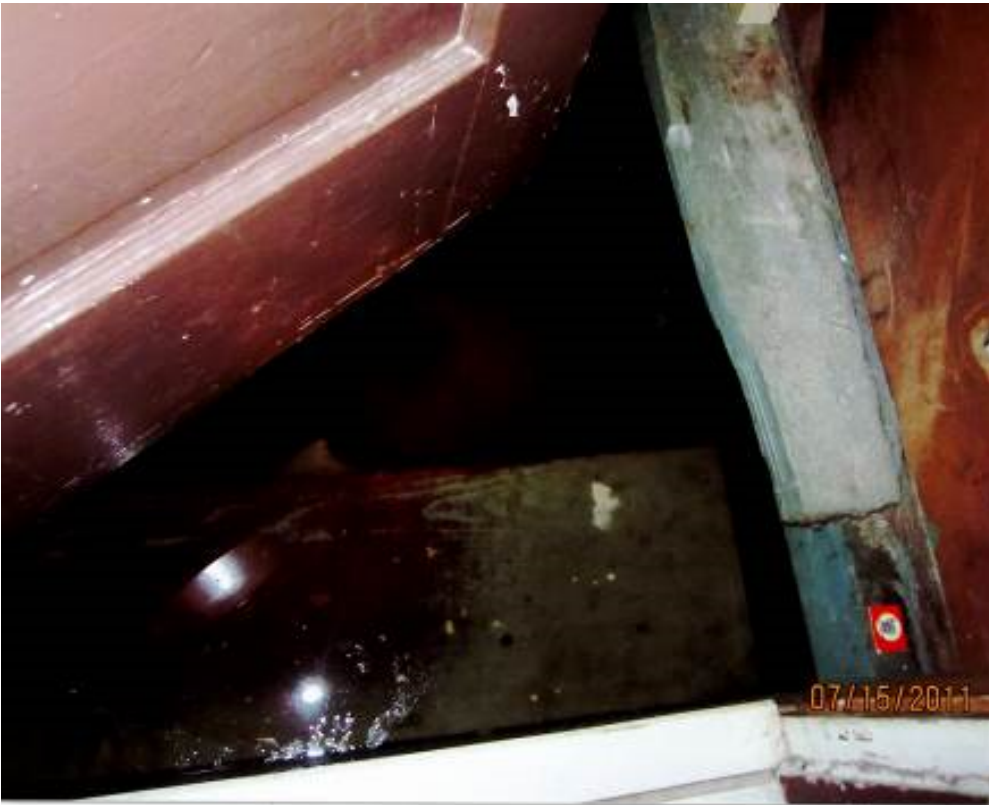
Water entering home from garage
